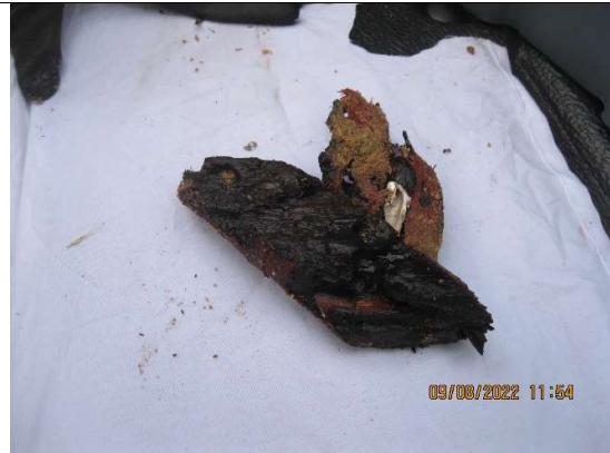
Photo 10: Core from Pier 10. White head of dead Teredo can be seen in the cavity created by the borer
