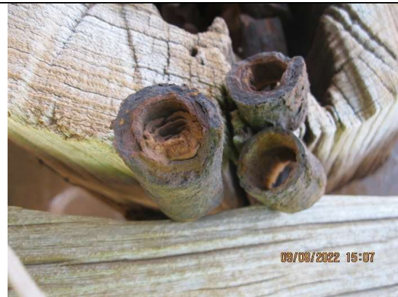
Photo 22: Unusual corrosion mechanism of bolt
