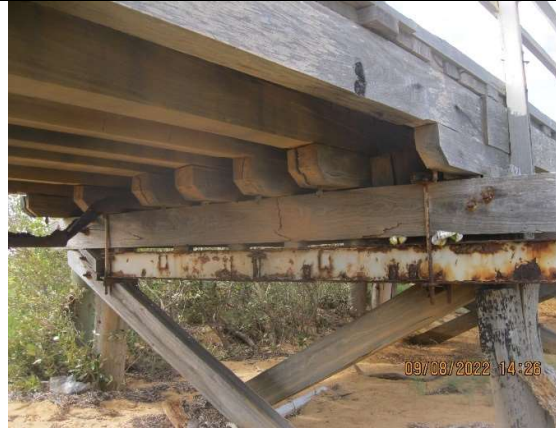
Photo 14: Cracked crosshead strengthened by underslung steel member
