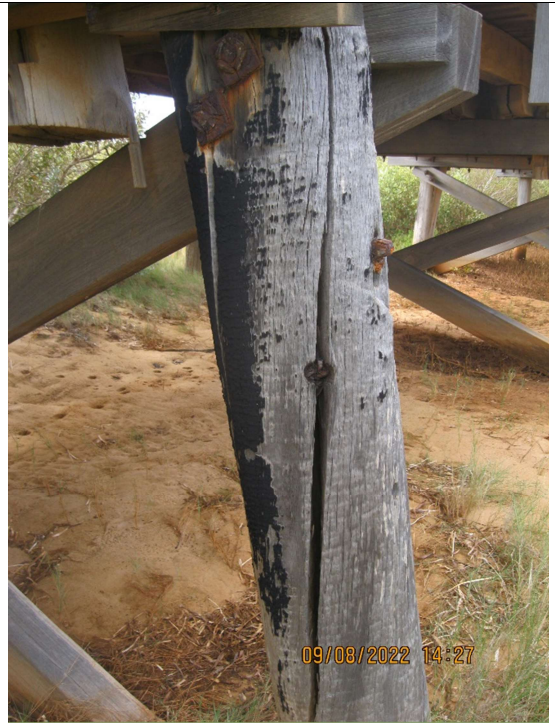
Photo 4: Pile replaced circa 1950 showing remnant black pile treatment. Remains of original pile still attached to crosshead.
