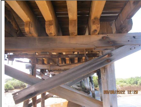
Photo 15: Incomplete cross bracing and cracked crosshead
