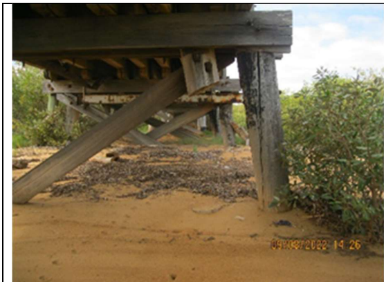
Photo 6: Replaced pile showing black remnants of pile treatment
