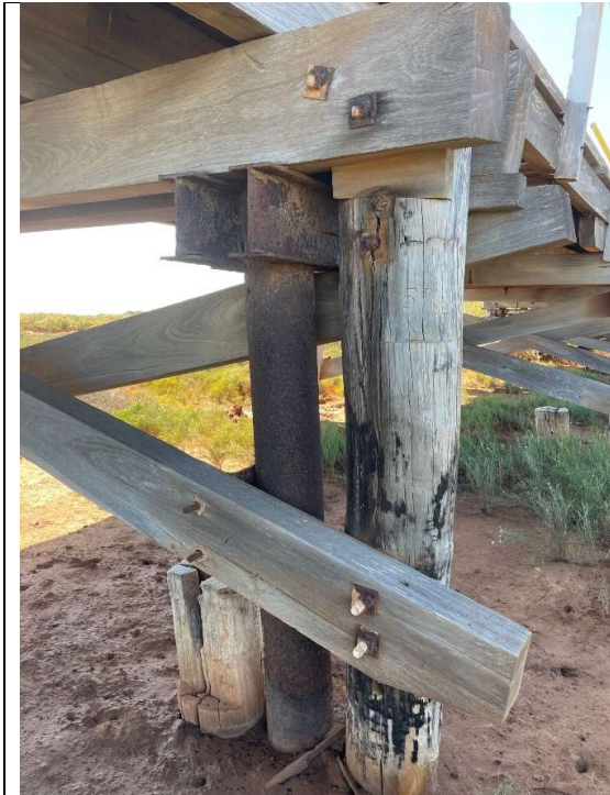
Photo 3: Pile replaced circa 1950 showing remnant black pile "charred and tarred" treatment
