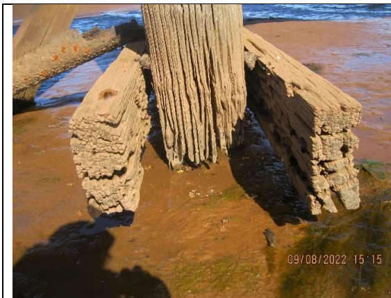
Photo 17: Rotted lower waler and pile
