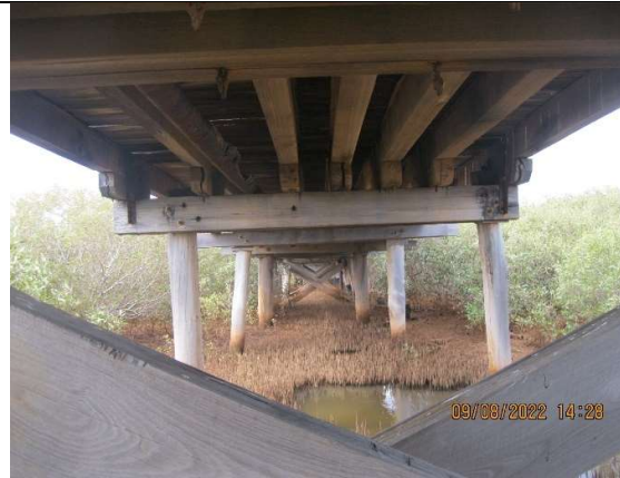
Photo 16: No cross bracing in 3 consecutive bays
