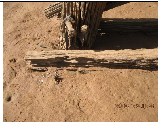
Photo 18: Disconnected lower waler
