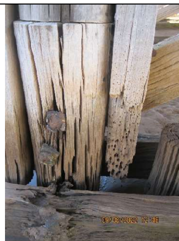
Photo 12: Split original pile which has been spliced with new upper section. Splicing supports either side showing evidence of marine borers.
