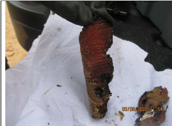
Photo 9: Limited core extracted from Pier 110 showing evidence of marine borers
