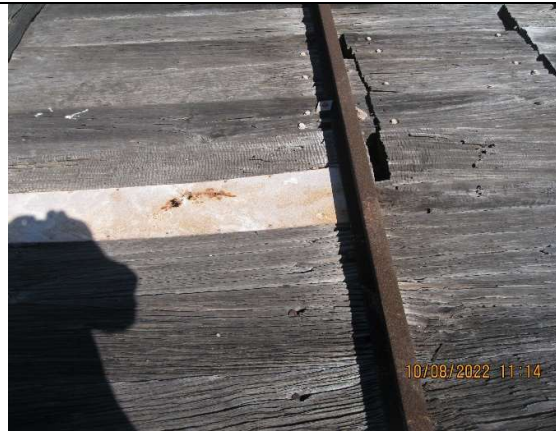
Photo 25: Weathered deck boards
