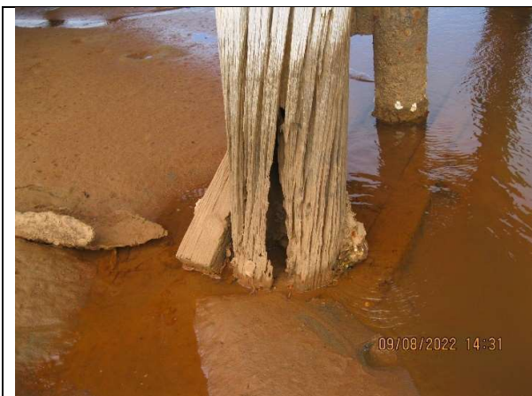
Photo 11: Split and rotted pile in intertidal zone - replacement steel pile alongside is corroded.
