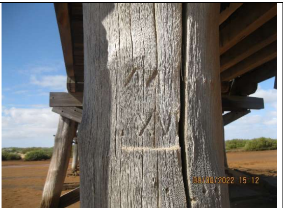
Photo 7: Replaced pile showing markings - 44 indicates year of replacement (1944) and roman numerals XXVI indicates length of pile at 26 feet.
