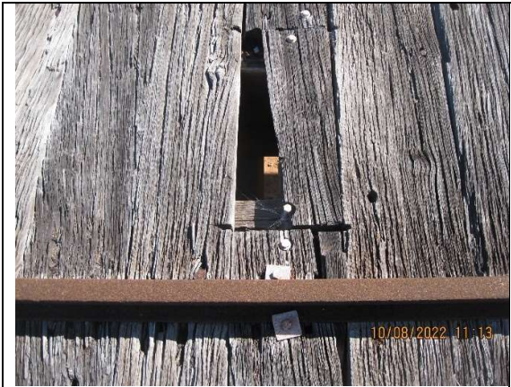
Photo 24: Split and weathered deck boards
