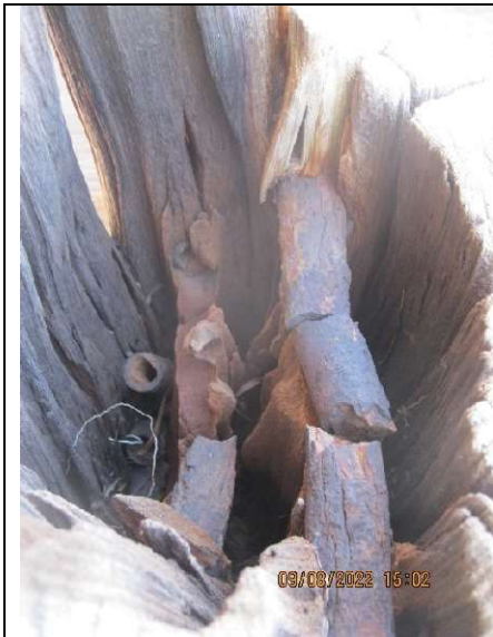
Photo 21: Corroded bolts inside a rotted cut off pile
