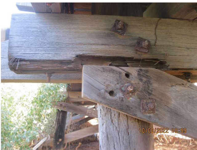
Photo 23: Termite damage to crosshead
