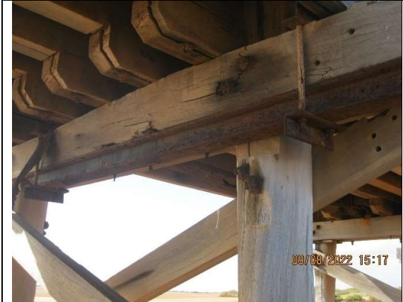
Photo 13: Cracked crosshead strengthened by underslung steel member
